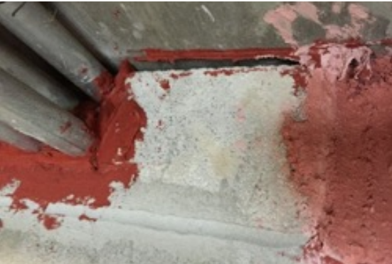
Fig. 35: Cracked sealant coating
