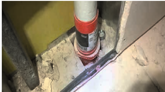
Fig. 17: Hilti CP 680 sleeve not cast into concrete
