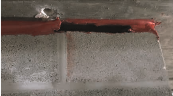
Fig. 29: Gap in application
