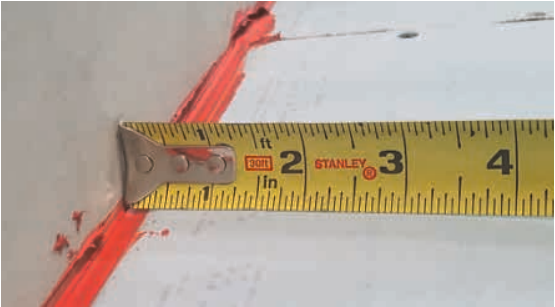
Fig. 30: Inadequate width of the sealant/gap
