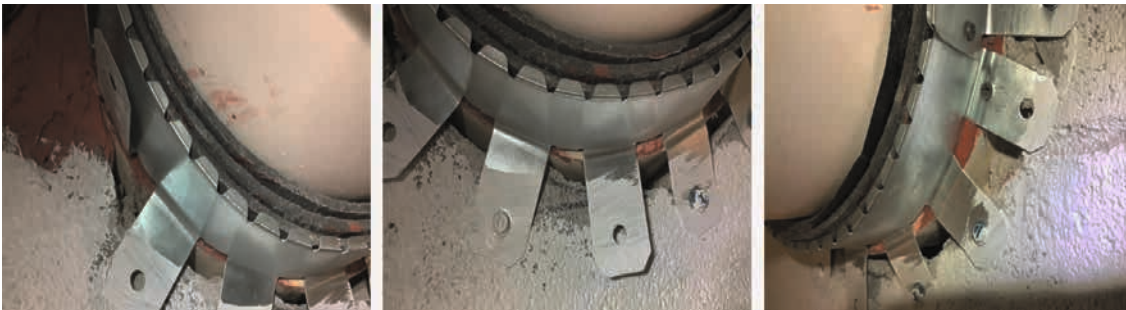
Fig. 18: Gaps in opening exist
