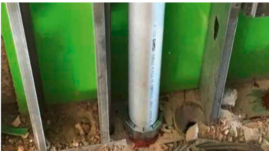
Fig. 19: Incorrect installation of collar installed on top side of floor
