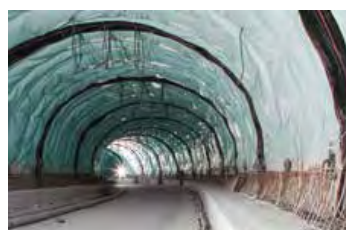
a) Road tunnels are highly corrosive environments
