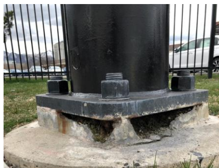
Figure 1. Poorly installed dry-packed grout pad
